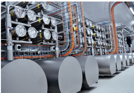
A RO process requires substantial pressure that is built by a row of heavy pump equipment by Alfa Laval (photo: IDM)
