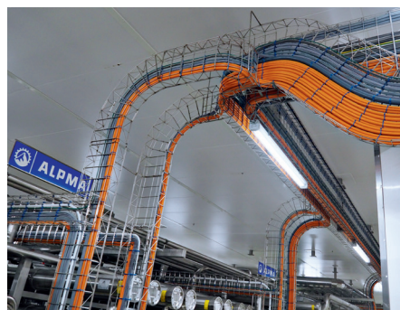
A single look onto the wiring shows how much care was taken during installation of the RO plant (photo: IDM)
