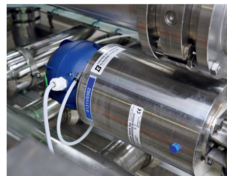
A single look onto the wiring shows how much care was taken during installation of the RO plant (photo: IDM)
