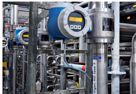
Peripheral equipment such as sensors was supplied by renowned manufactures such as Endress + Hauser (photo: IDM)
