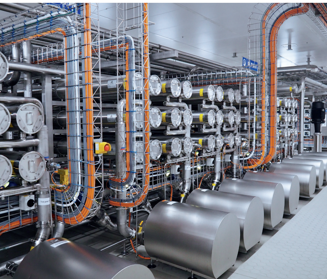
The Gerkesklooster RO plant type ALPMA RO HighTS has a membrane surface of over 10,000 sqm (photo: IDM)
