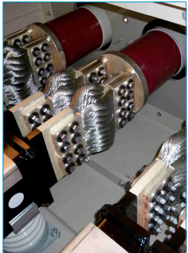
5000A generator connection
